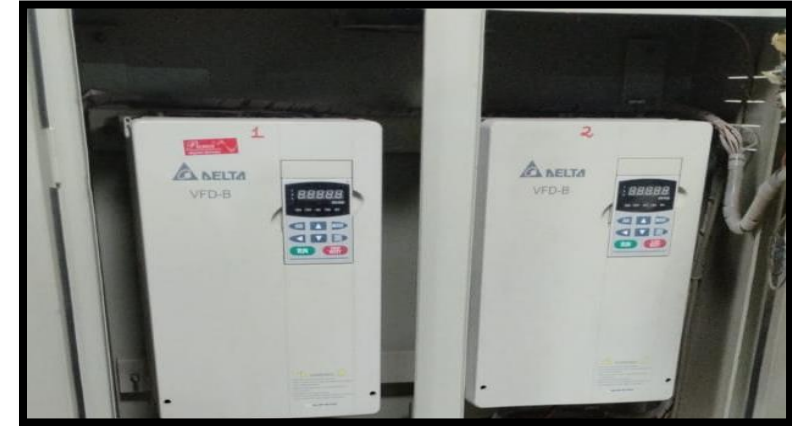
02 VFD on Boiler Blower Motors
