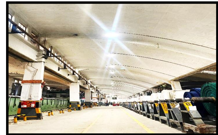
Installed Day Light Saving Sensors
